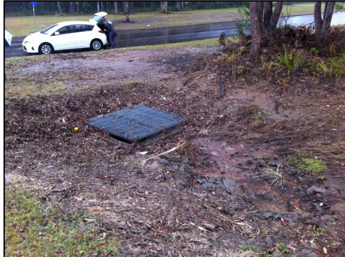
Figure 6-9 Erosion at Drainage Inlet Upstream of Coachwood Drive
